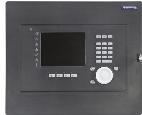
Gabinete com painel operacional
