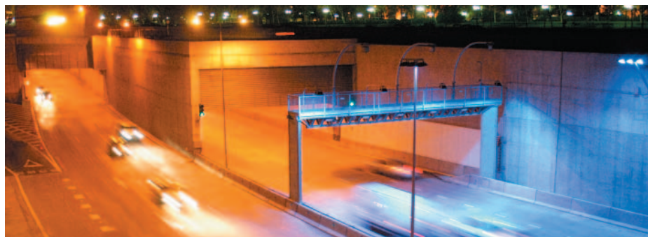
Tried and proven: tunnels in Chile's capital city Santiago de Chile are protected from fire thanks to SecuriSens® TSC 515 temperature sensor cable.
